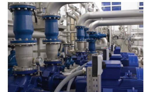
• The city concentrated water supply
