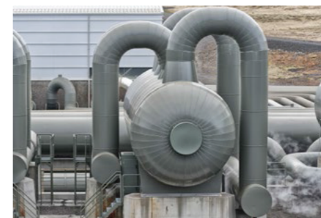
• the water supply pump station
